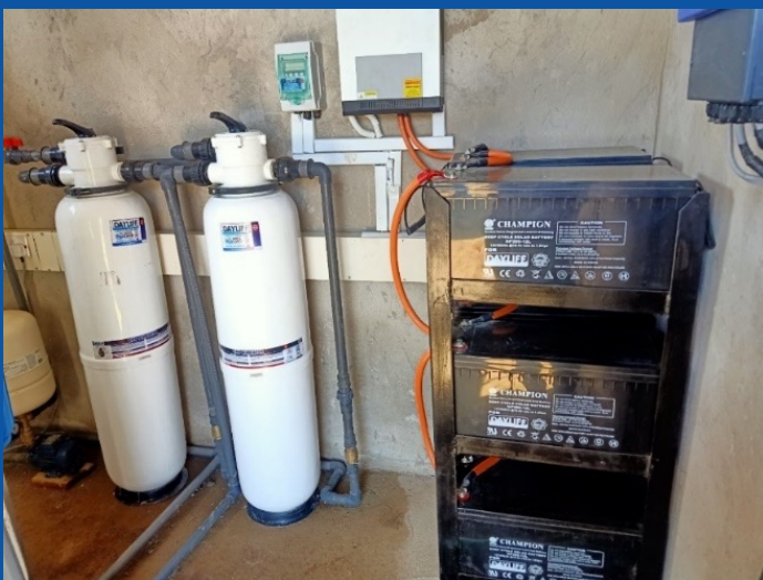
Water purification system
