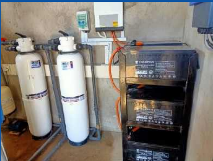
Water purification system
